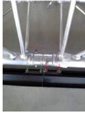
(b) Connecting joints of the rail.
